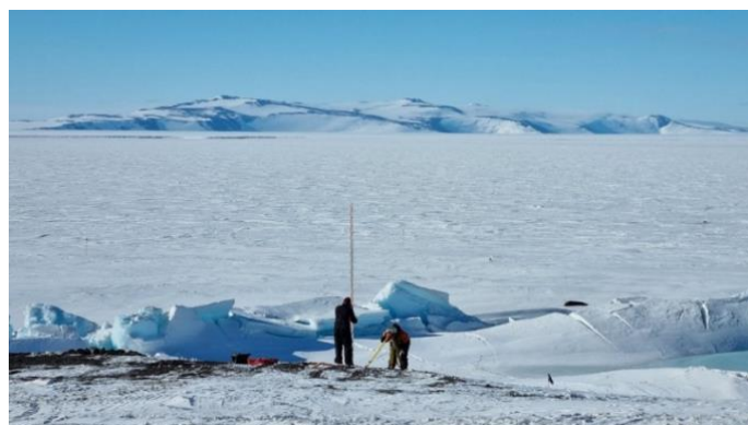
Precise levelling undertaken to check the stability of the site where the historic Trans-Antarctic Expedition/International Geophysical Year hut, at Pram Point, November 2021 Photo: Toitū Te Whenua LINZ
